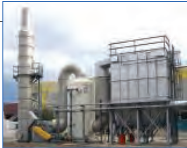
FIGURE 2. This installation includes a dust collector for ash and particulate matter, quench to cool combustion gases, a vertical packed tower for SO 2 removal and a stack and fan for ventilation. It represents a total solution for SO 2 and pollution abatement
